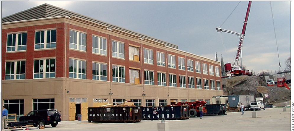
One Brigham Circle, a $45 million mixed-use project in Boston's Mission Hill section, will open most of its stores this month.
